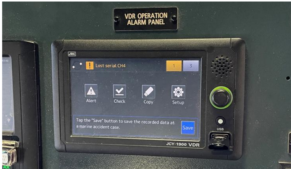
Figure 6. Photo of the JCY-1900 Operation Panel Unit mounted on the Dali's bridge console.
