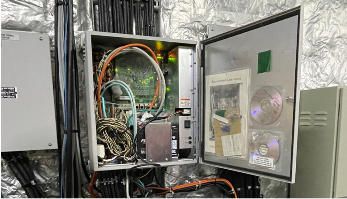
Figure 2. Photo of VDR cabinet mounted in an electrical room below the bridge on the Dali .
